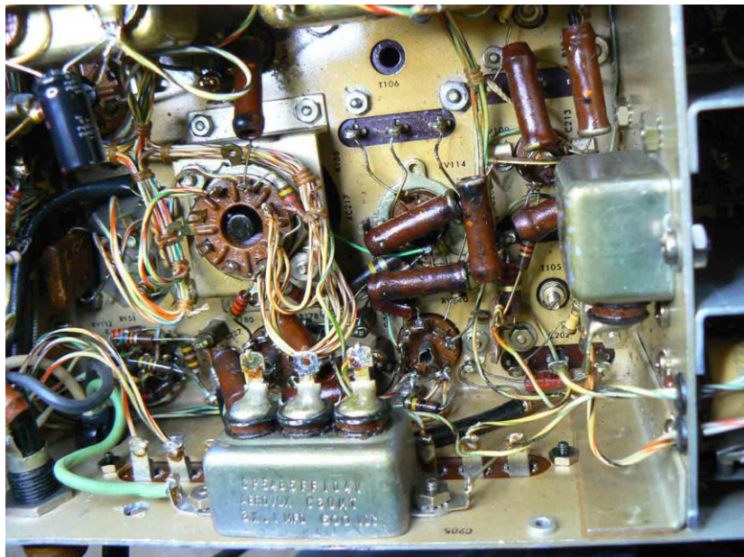
Fig. 4 –The wire has been removed from C205B (the middle terminal on the triple “bathtub” capacitor near bottom center). You can also see the green wire from the PD3, which has been routed beside the large filter capacitor (in the octal socket) to V114, pin 5.
